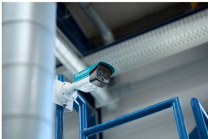
Caption 2: With “Hotspot Monitoring,” Vecoplan is closing a gap in early fire detection at recycling facilities.
