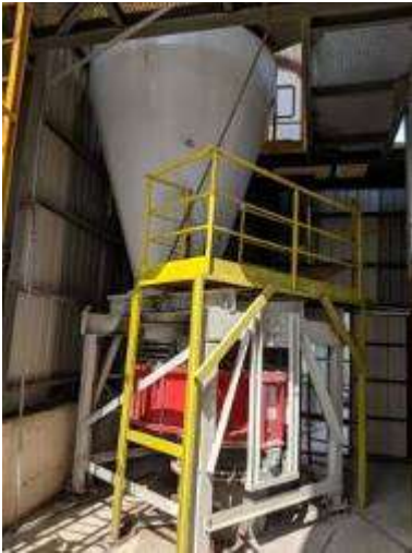
Image 6: The gravimetric dosing system ensures constant, uniform feeding of the preheater.
