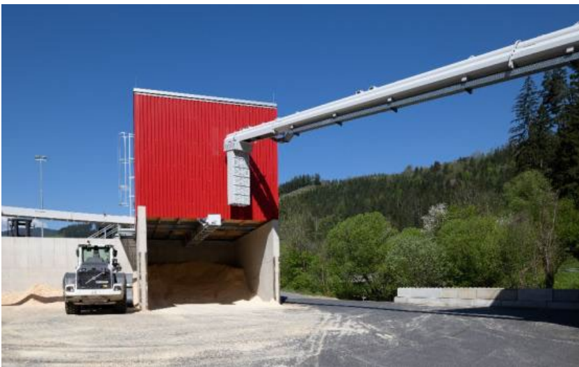
Photo 5: The fine wood chips are conveyed via the VRF 500 P pipe belt conveyor system to the VSS 6000 vibrating separator above the sawdust boxes.
