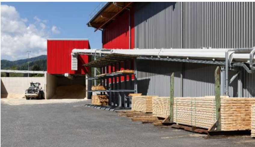
Photo 3: The VRF 500 P was specially developed for the clean and quiet transport of bulk materials over long distances and is used by Schaffer on an 80-meter route throughout the entire yard.
