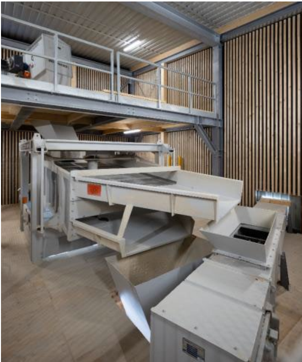
Photo 4: The intelligent screening system with the VSS 6000 vibrating separator ensures the effective screening of the wood chips.
