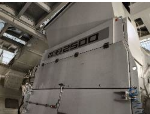
Photo 9: For the secondary shredding process, the MBS plant relies on the VEZ 2500, which was specially designed for the production of substitute fuels.
