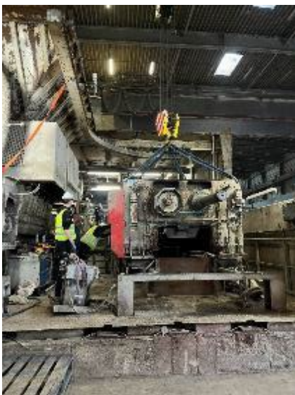
Photo 6: The VVZ 2500 was refurbished in the autumn of 2024, as part of a maintenance project.
