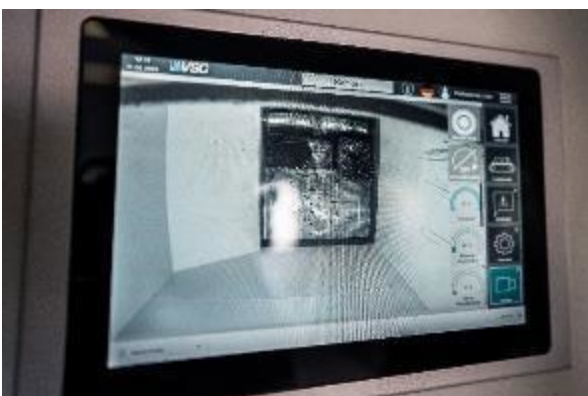
Photo 2: A camera gives the plant manager a complete view of the sensitive areas.
