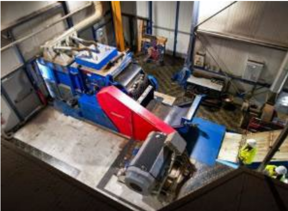
Photo 3: Material is fed to the system outdoors via a conveyor belt. The shredding itself takes place indoors for noise reduction.
