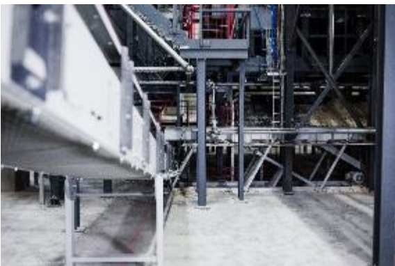
Photo 3: The conveyor system transports the material to the individual stations.
