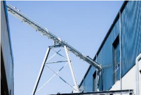
Photo 7: The Vecobelt transports the material across the yard to the storage boxes and the screening station and then to pellet processing.
