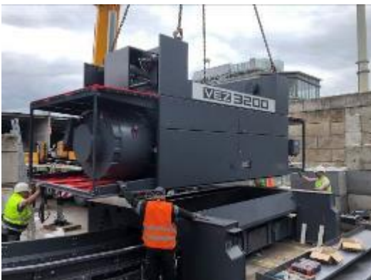
Photo 5: Vecoplan extended the system by installing an additional single-shaft pre-shredder from the VEZ 3200 series which generates material with a particle size of less than 250 millimetres.
